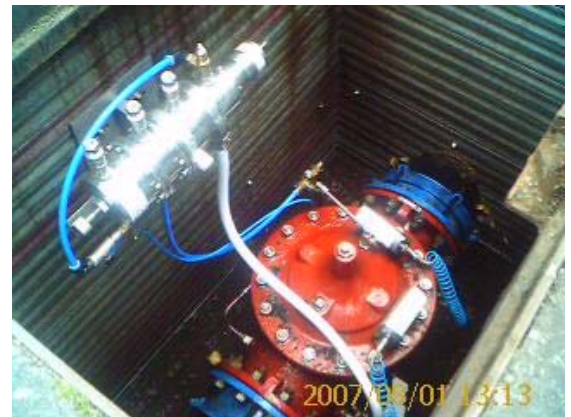
An Aquai-Mod® installed in a typical PRV chamber
